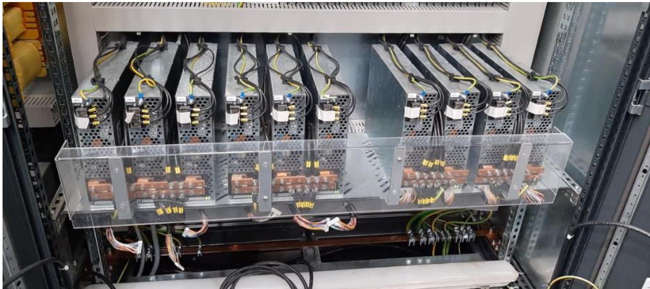
Figure shows 10 x Power units installed in equipment
